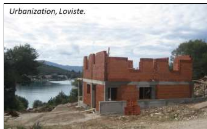
Figure 54: House building in Loviste in front of the sea (photography: M. Graziella)
